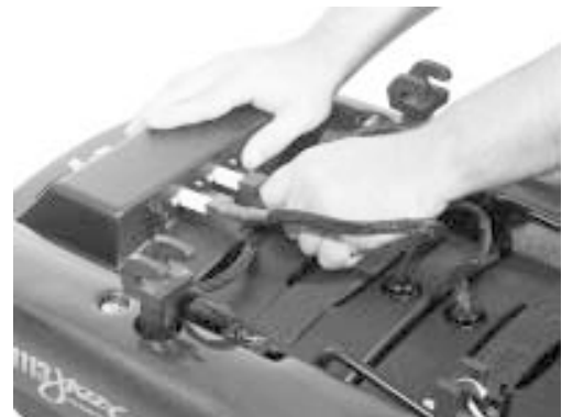
Figure 34. Disconnecting Battery Box Connections
