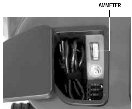
Figure 38. Utility Tray (Uncovered)
